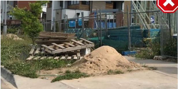
EXAMPLE OF POORLY MANAGED STOCKPILE
