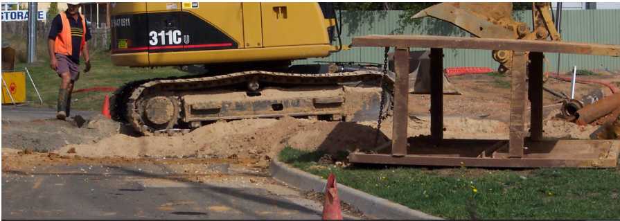
IMAGE 4: INAPPROPRIATE CONTROL MEASURES
