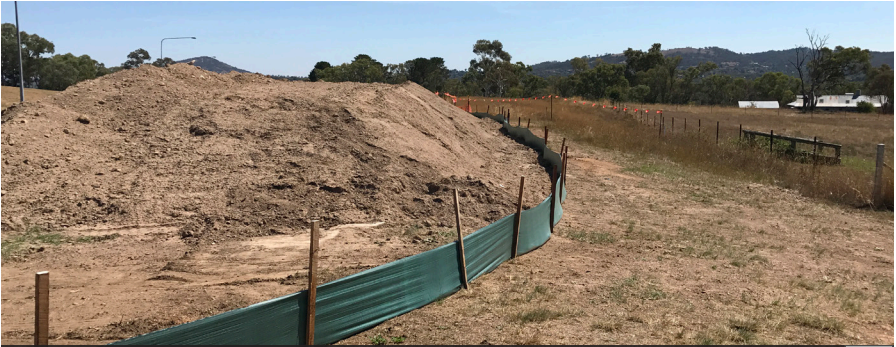
IMAGE 10: SEDIMENT FENCE AROUND STOCKPILE
