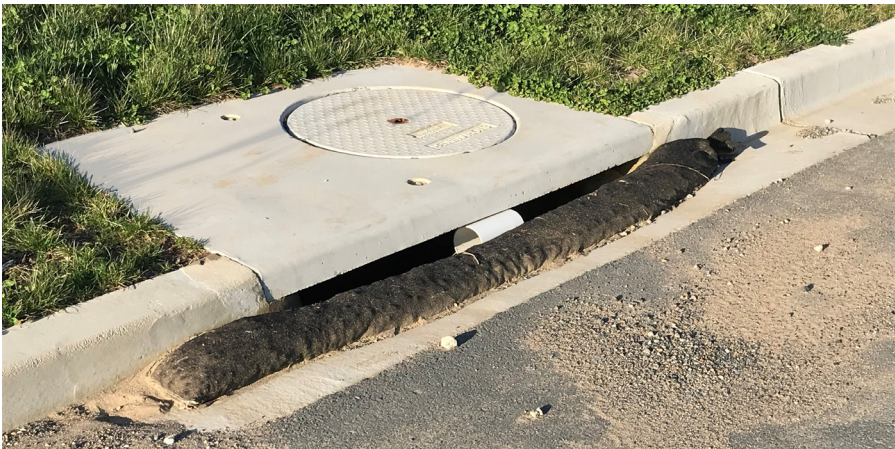
IMAGE 2: KERB INLET CONTROL WITH GRAVEL WRAPPED IN NETTING AND GEOTEXTILE FABRIC
