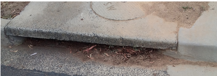
IMAGE 5: POLLUTION ENTERING STORMWATER DRAIN
