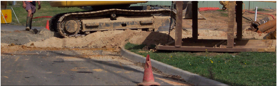
IMAGE 7: UNSATISFACTORY STABILISATION HAS RESULTED IN SEDIMENT LEAVING THE SITE
